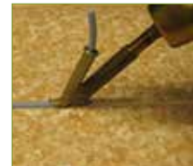
2- WELD: Using a welding gun and nozzle suitable for solder joint (pinched fast nozzle for long lengths, corner finish nozzle for finishes, ...)
