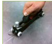
1- GROOVE: Using a tool for manual grooving or electrical grooving, for opening the joints from 3 to 4 mm.
