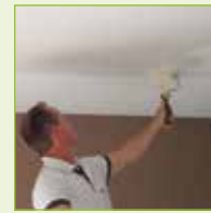
glue on the ceiling.
